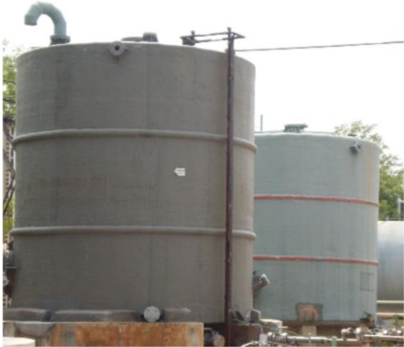
PVC FRP Tanks
